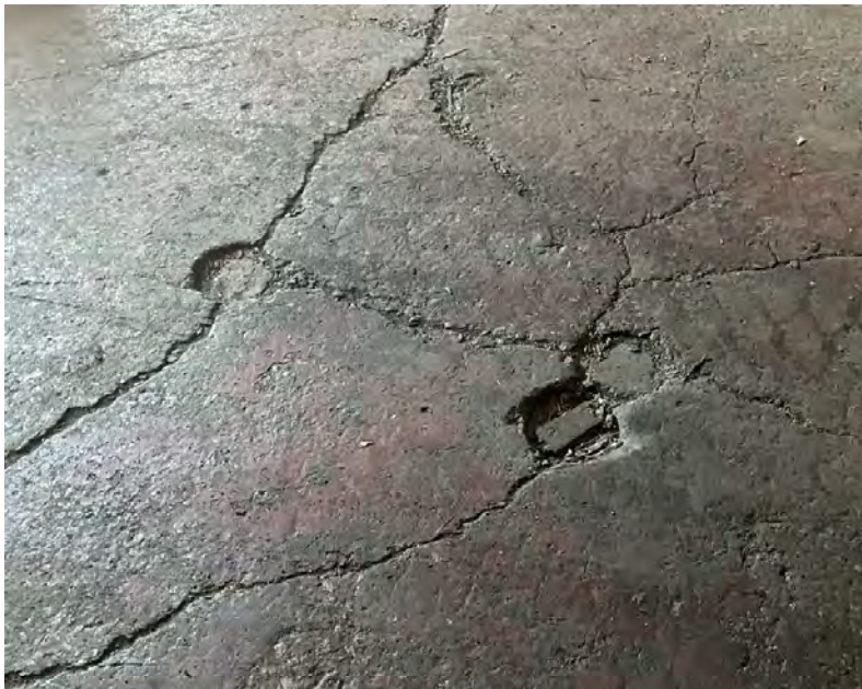
Photo 2: Interior Floor – view of the floor in the northwest portion of the building adjacent to the loading dock area with cracks and holes.
