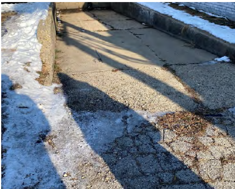
Photo 6: Exterior Paved Area – loading dock and adjacent asphalt pavement have cracks.
