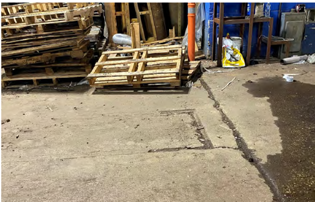
Photo 4: Interior Floor – view to the east of the floor in the southeast portion of the building with cracks needing repair.
