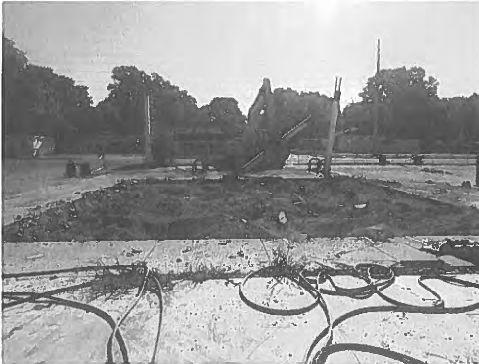
Date: 8/30/2022 Time: 9:29am Direction: E Photo by: Robert Mileur Exposure #: 001 Comments: Tank field being uncovered for tank removal.
