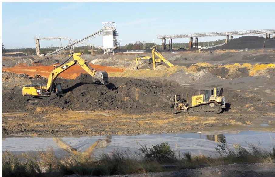
Photograph of removal process taken during visit to the Wateree Station in South Carolina.
