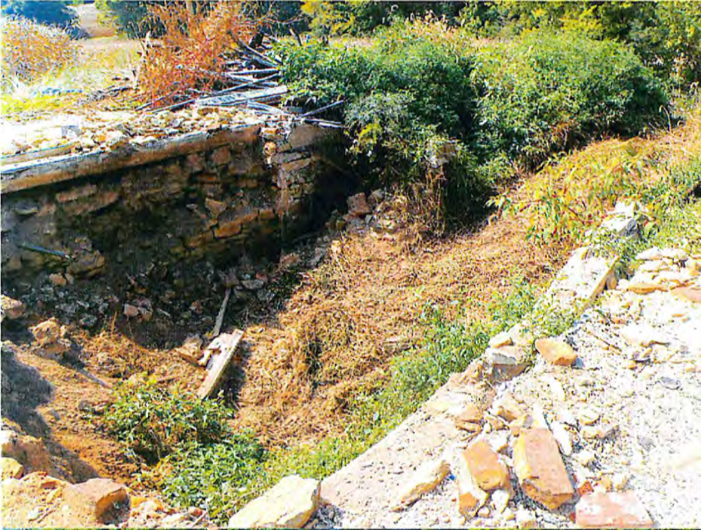
Date: 10/01/2014 Time: 12:30 PM Direction: S Photo by: Zappa Exposure #:001 Comments: Demolition debris that needs to be cleaned up and the foundation was dug up.
