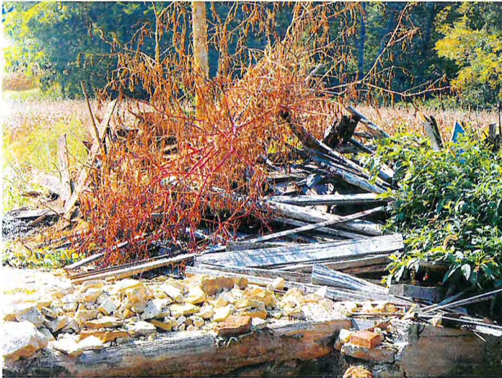
Date: 10/01/2014 Time: 12:34 PM Direction: SE Photo by: Zappa Exposure #:003 Comments: A wide view of the demolition debris that has been left behind.
