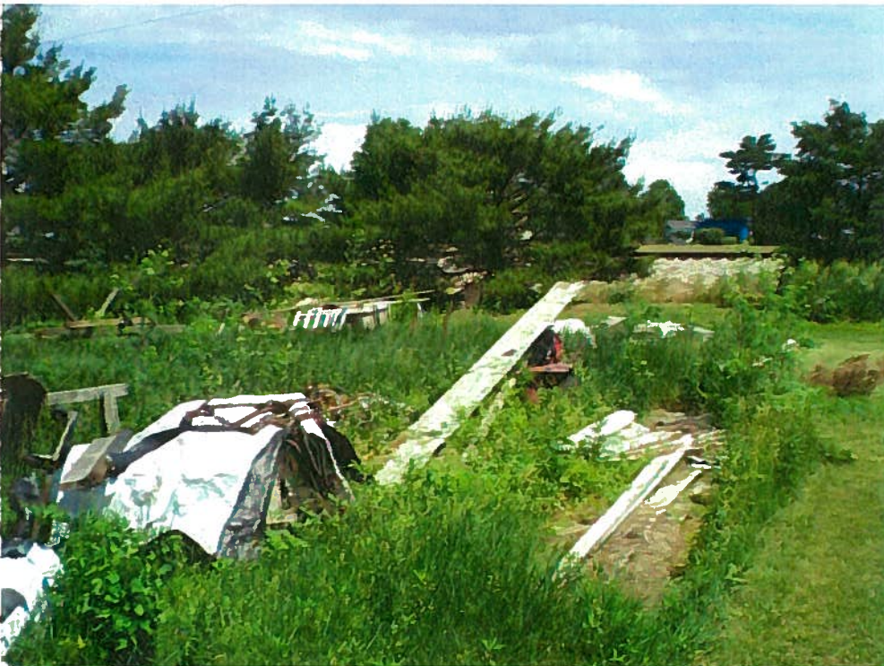
Date: June 1, 2011 Time: 11:49 AM Direction: North Photo by: W Zierath Exposure #: 016 Comments: The northwest part of the site showing scattered demolition waste, old pallets, scattered scrap metal and other junk
