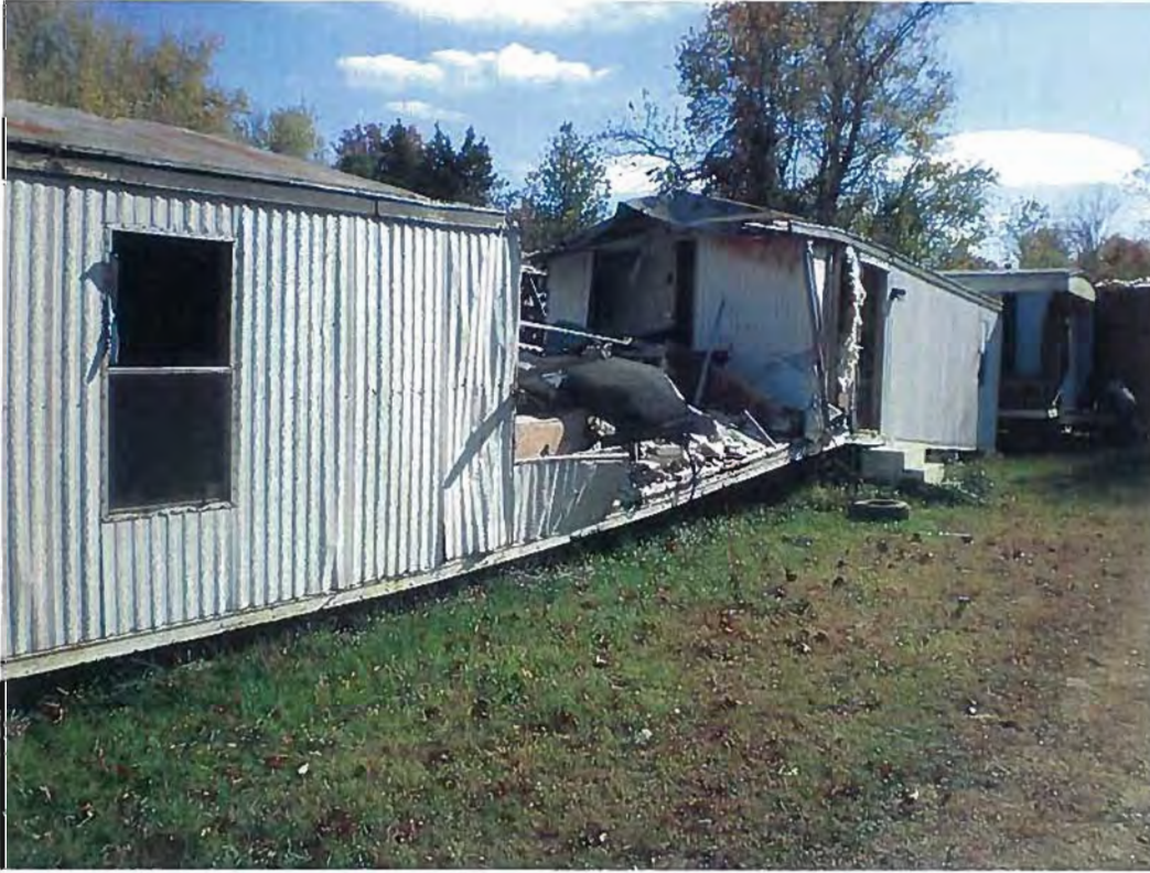
Date: 10/28/2010 Time: 2:00-2:30 PM Direction: Southeast Photo by: M. Stevenson Exposure #: 007 Comments: Mobile home with center section missing wall and roof sections.
