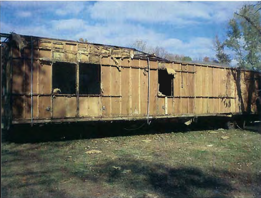
Date: 10/28/2010 Time: 2:00-2:30 PM Direction: Southeast Photo by: M. Stevenson Exposure #: 008 Comments: Mobile home being demolished.
