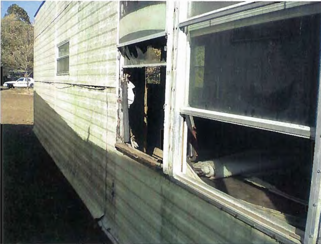
Date: 10/28/2010 Time: 2:00-2:30 PM Direction: North Photo by: M. Stevenson Exposure #: 019 Comments: Mobile home missing windows.
