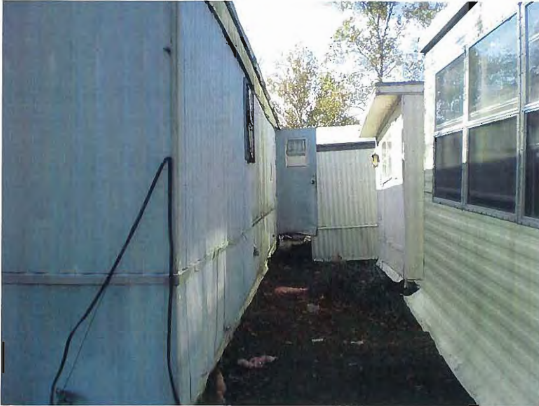
Date: 10/28/2010 Time: 2:00-2:30 PM Direction: West Photo by: M. Stevenson Exposure #: 015 Comments: Mobile homes in various stages of demolition.
