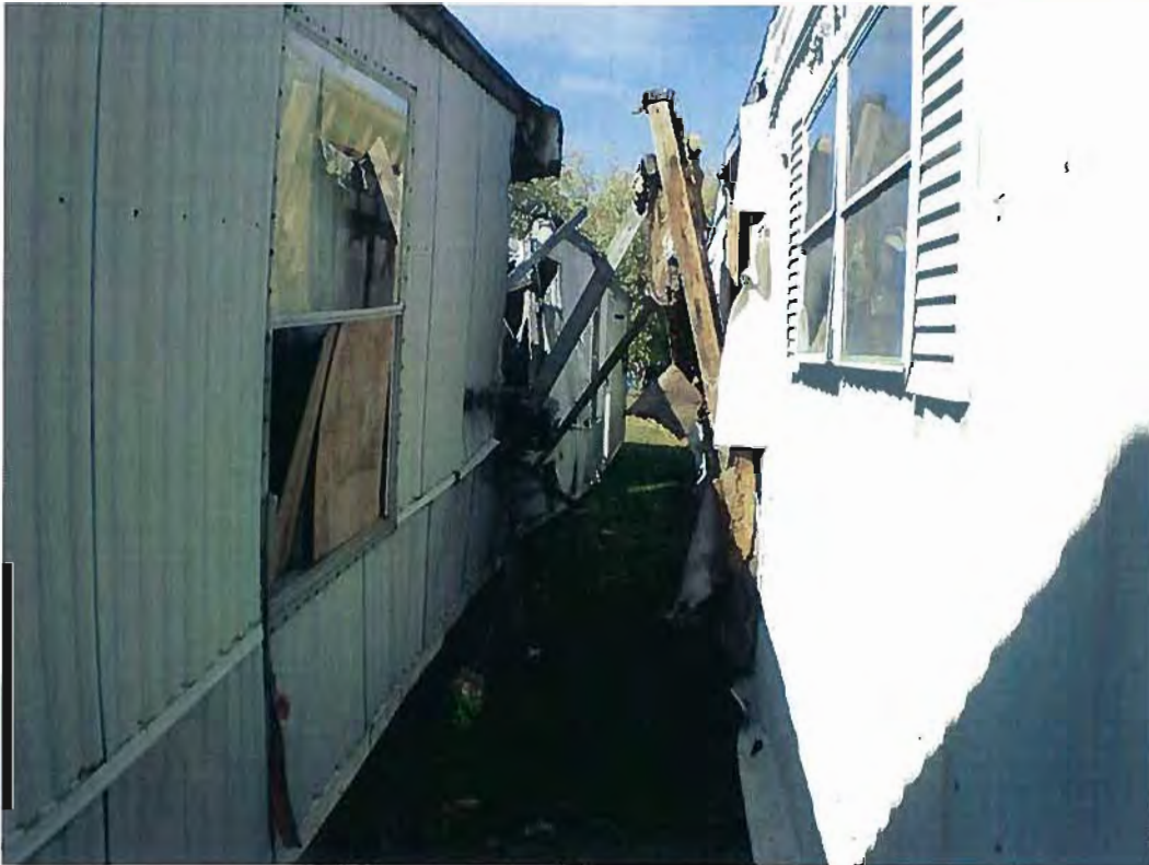
Date: 10/28/2010 Time: 2:00-2:30 PM Direction: North Photo by: M. Stevenson Exposure #: 018 Comments: Mobile homes in various stages of demolition.
