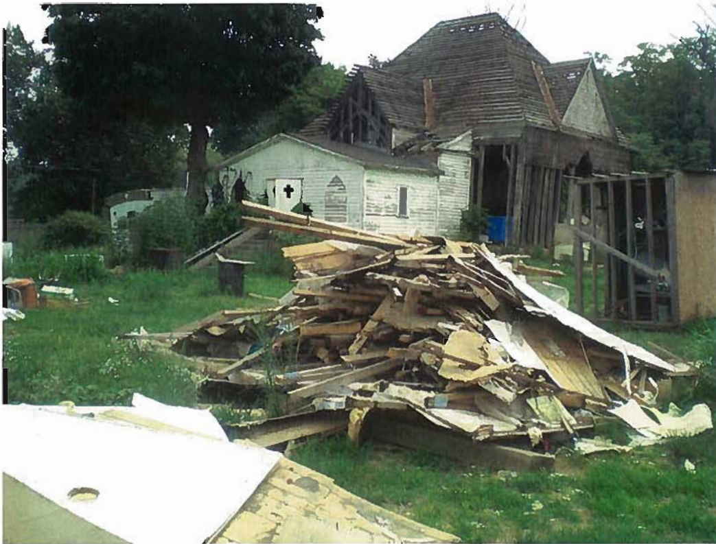
Date: August 9, 2010 Time: 10:56 Direction: NE Photo by: S. Townsend Exposure #: 011 Comments: Demolished mobile home wastes
