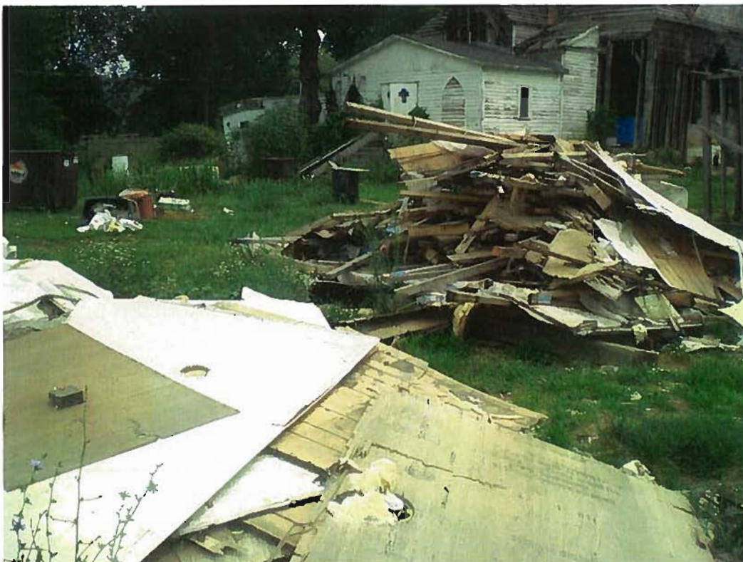
Date: August 9, 2010 Time: 10:56 Direction: NE Photo by: S. Townsend Exposure #: 012 Comments: Demolished mobile home wastes. Garbage in background.
