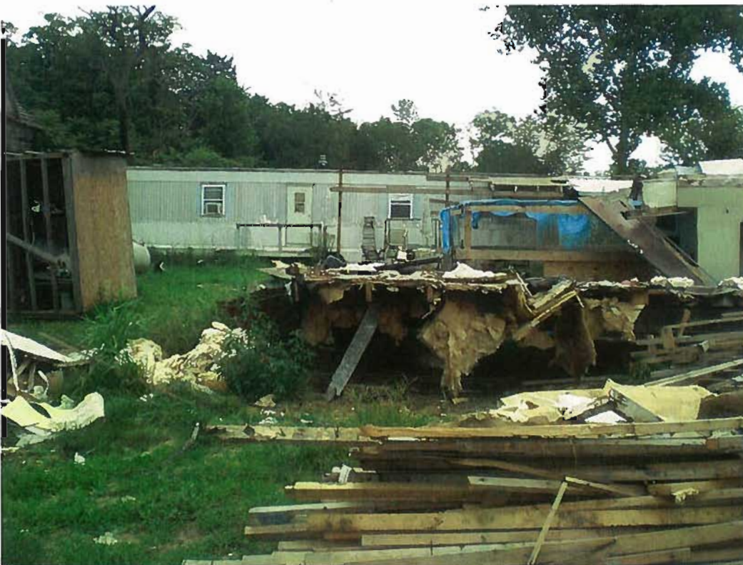
Date: August 9, 2010 Time: 10:56 Direction: E Photo by: S. Townsend Exposure #: 010 Comments: Demolished mobile home wastes, insulation, and scrap wood.
