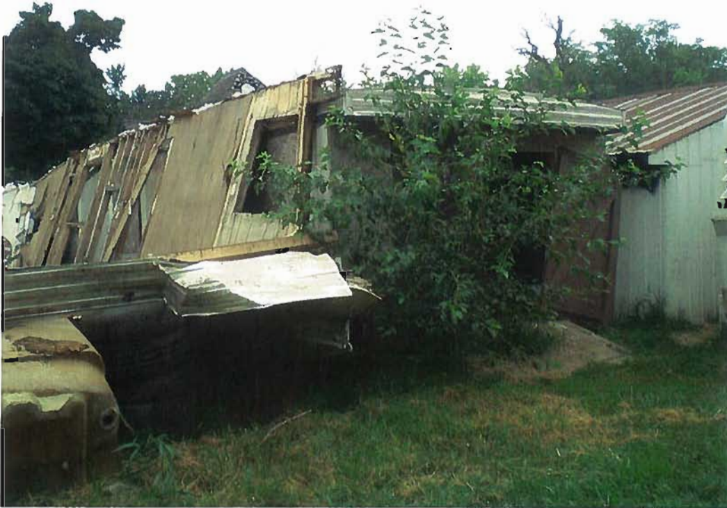
Date: August 9, 2010 Time: 10:53 Direction: N-NE Photo by: S. Townsend Exposure #: 005 Comments: Demolished mobile home wastes leaning against storage shed, and used tires under other wastes.
