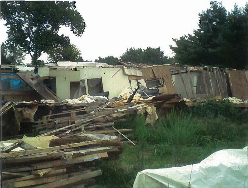
Date: August 9, 2010 Time: 10:56 Direction: E-SE Photo by: S. Townsend Exposure #: 009 Comments: Demolished mobile home wastes, including insulation, wood, and metal.
