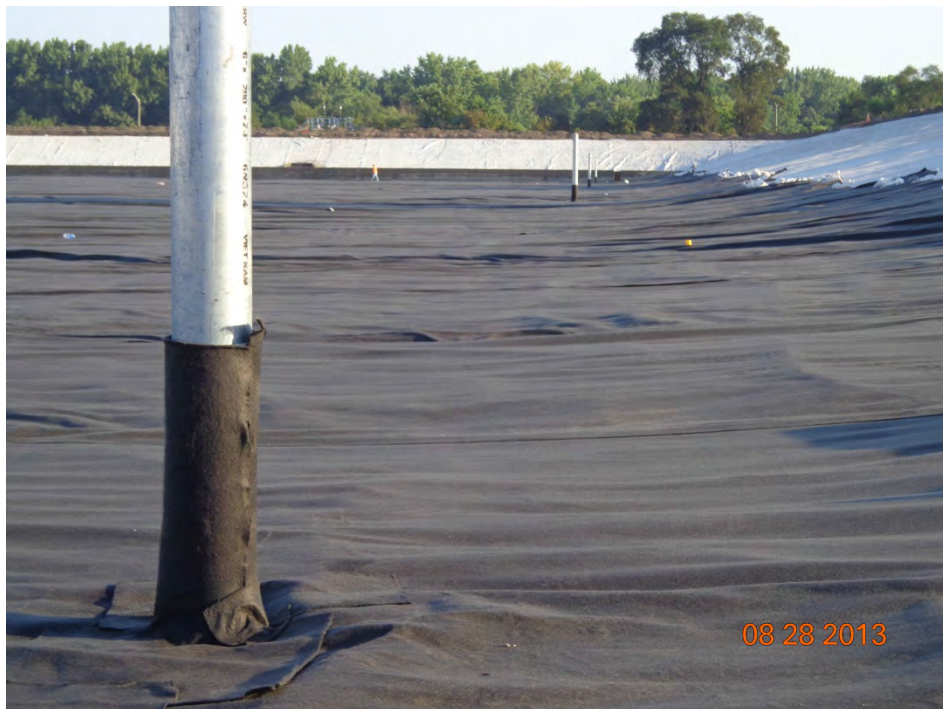
Geosynthetics liner penetration (looking north)
