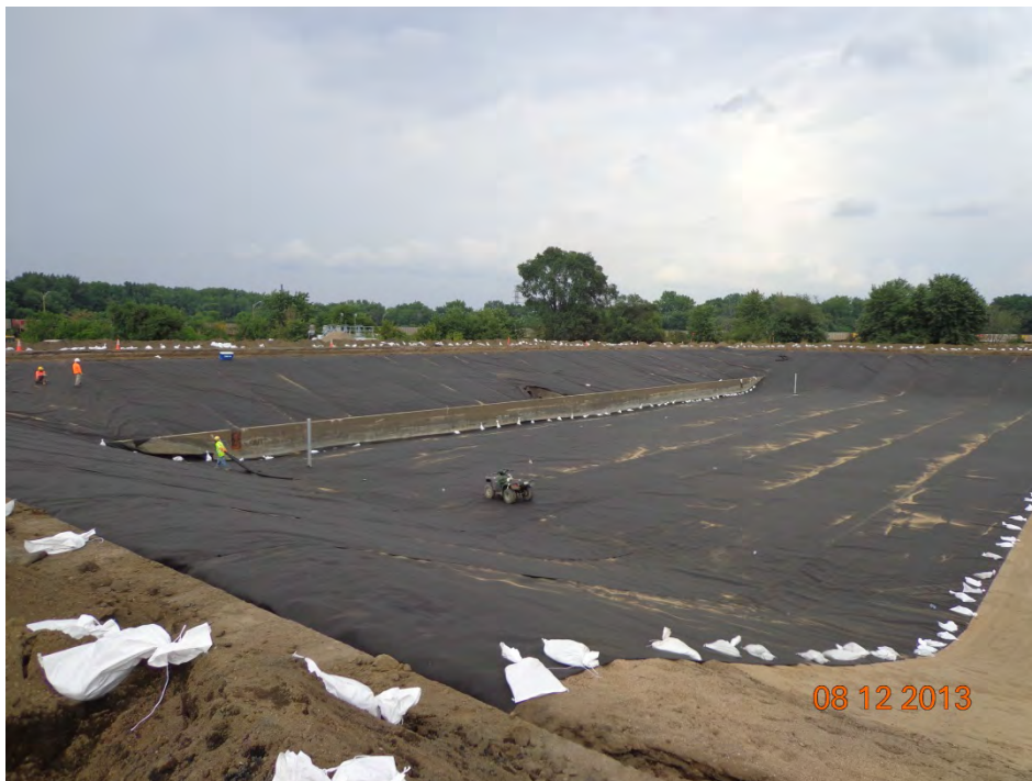
Extent of work completed on Day 1, south end of basin (looking southeast)
