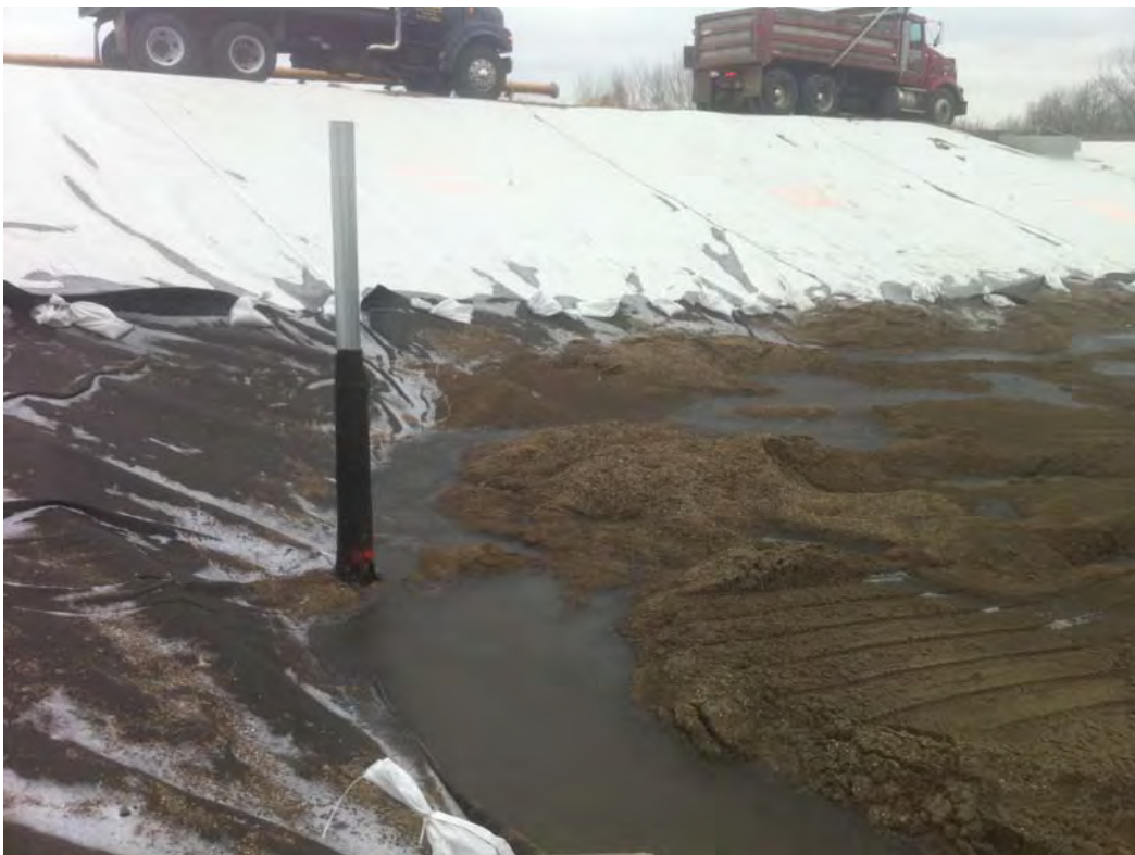
View of soft spots and ponding in the northern portion of the basin.
