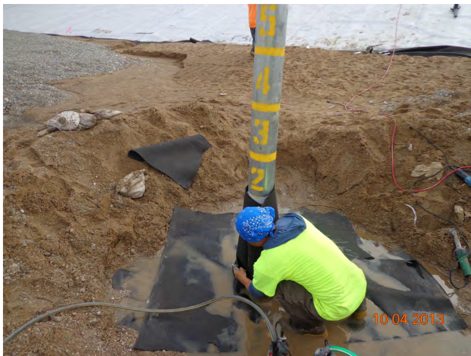
Installing the upper nonwoven geotextile over the geomembrane pipe boot (looking east)
