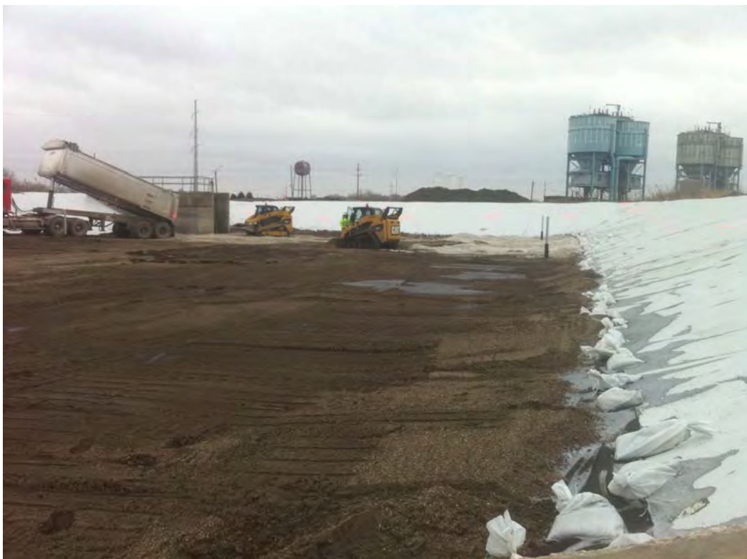
View of placement of warning layer in the southern portion of the basin.
