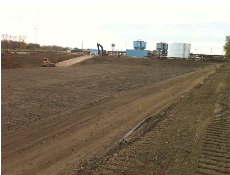
View of basin subgrade from the northwest corner of the basin facing southeast. Note concrete aprons and hypalon removed.
