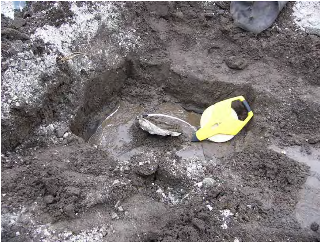
View of the uncovered leak in the bypass basin from the detection survey.
