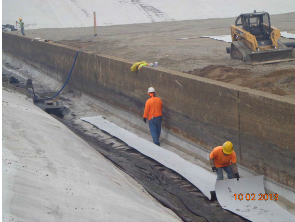
Geomembrane sections being added to the liner to provide slack for the transition between the basin floor and weir wall (looking southeast)
