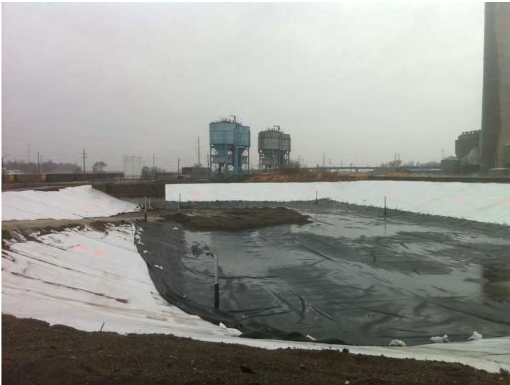
View of partially placed cushion layer in southern portion of the basin.
