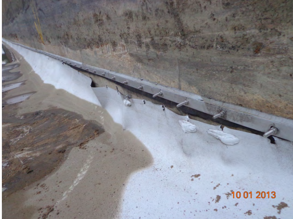
Section of the torn batten strip (looking southeast)
