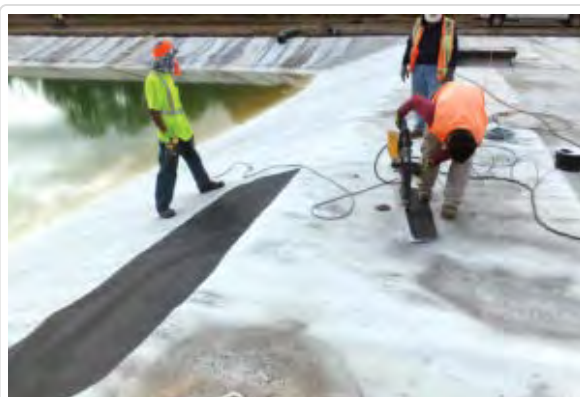
FIGURE 2 Patching a hole in pond liner where a sample was taken for testing in May 2014. The photograph shows trial weld being performed
