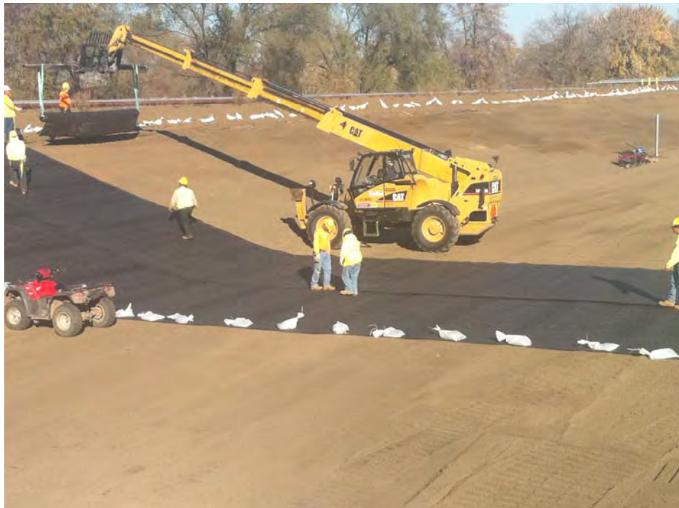
View of 16 oz geotextile being placed on the western slope and thermally bonded at the seams.
