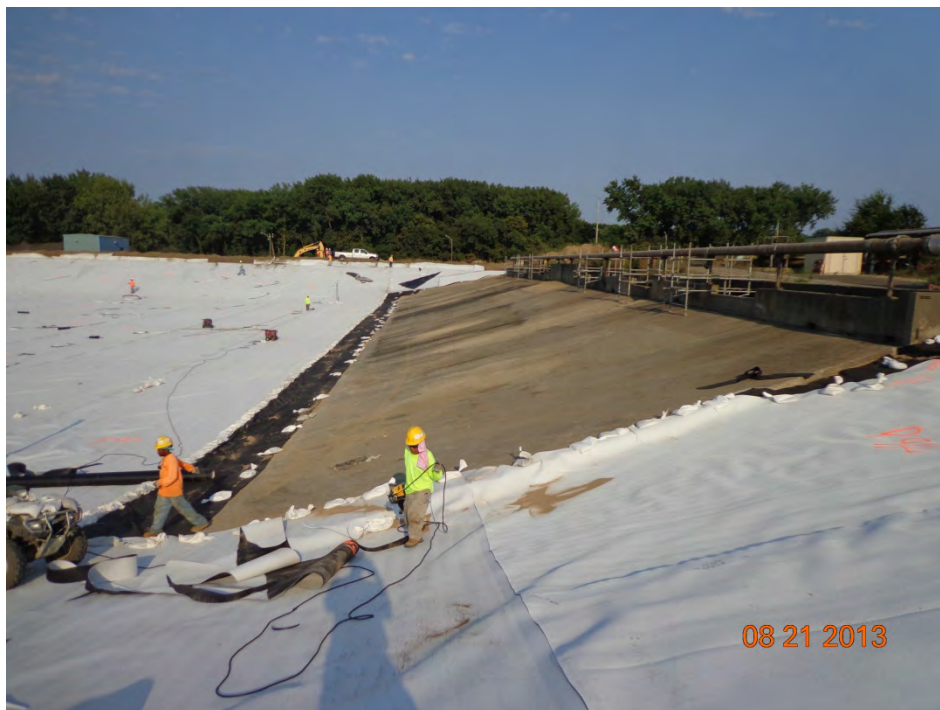
Extent of geosynthetics deployment on the south end of the basin (looking east)
