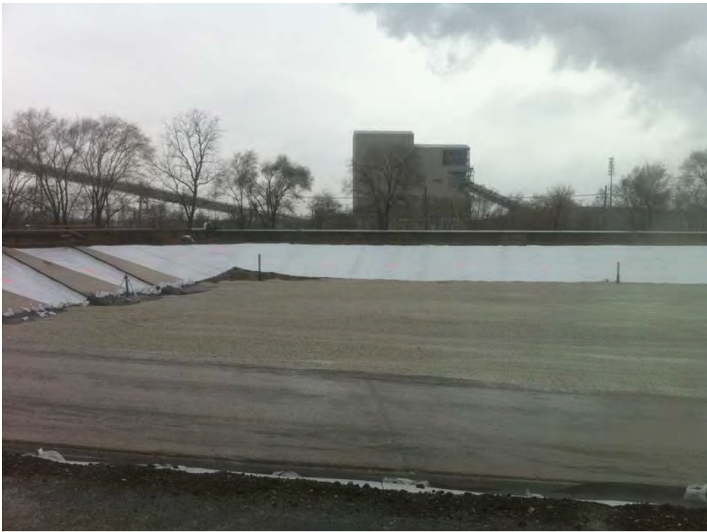
View of warning layer in the southern end of basin where additional cleanup and finishing is required.
